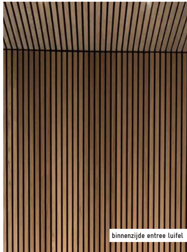
luifels in felsbanen
